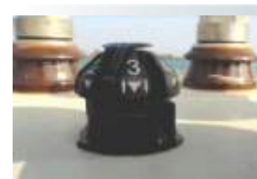
Off-Load Tap Changer
